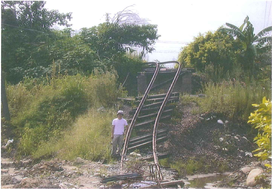
Figure 2. The earthquake rupture across the Chi-Chi railroad in the Mingjian , the eastern side shows a ground uplift of about 3 m.
